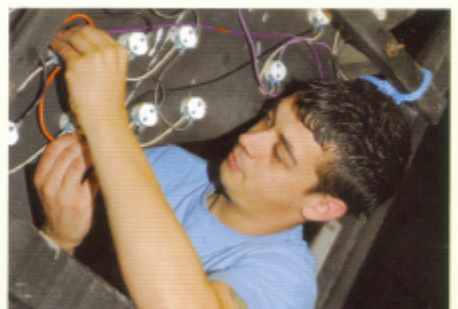
Electrician Daniel Doherty does some last-minute tweaking to one of the features
